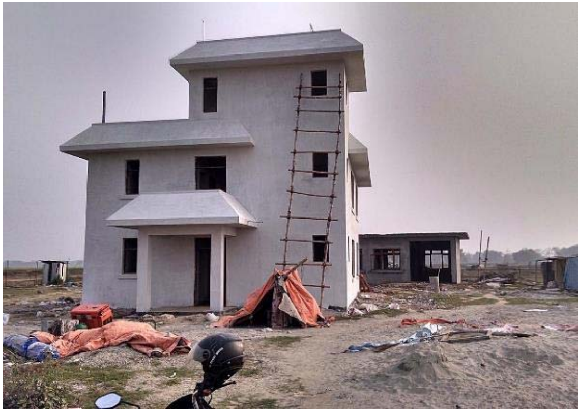
3. Office cum Lab Building WWTP, Jatuwa
