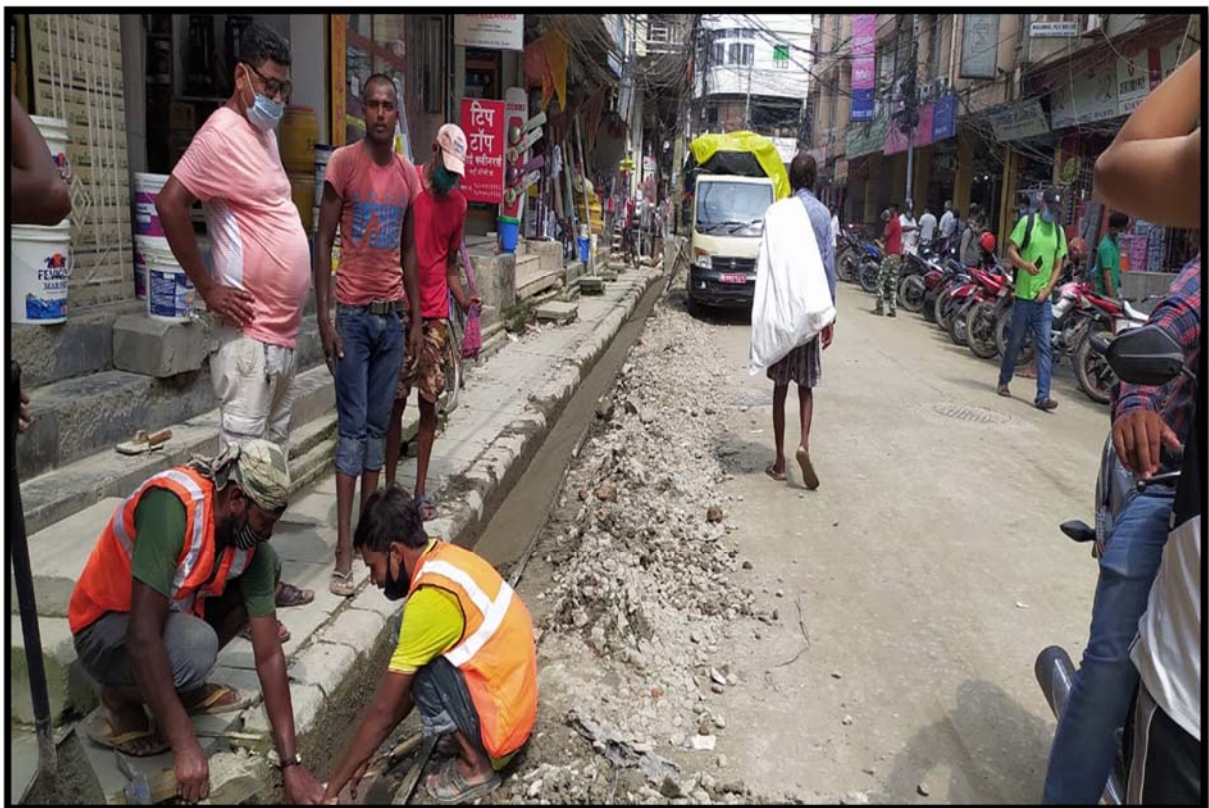
Teak drain at Hanuman Das Road
